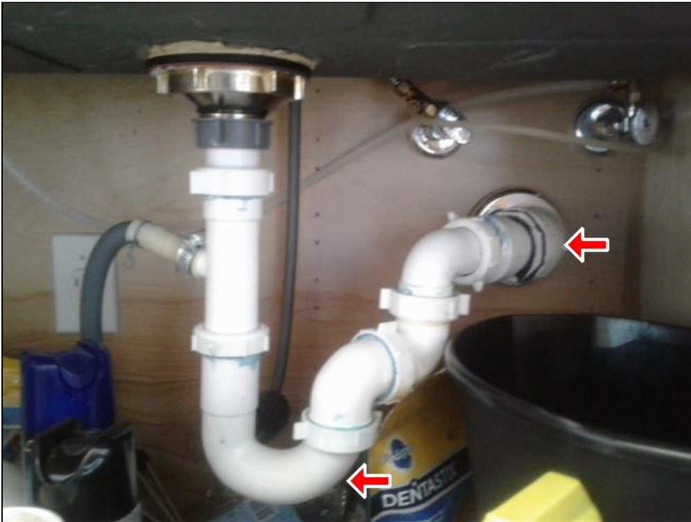
10.21 Item 1(Picture) Sink trap weir set too far below drain line
