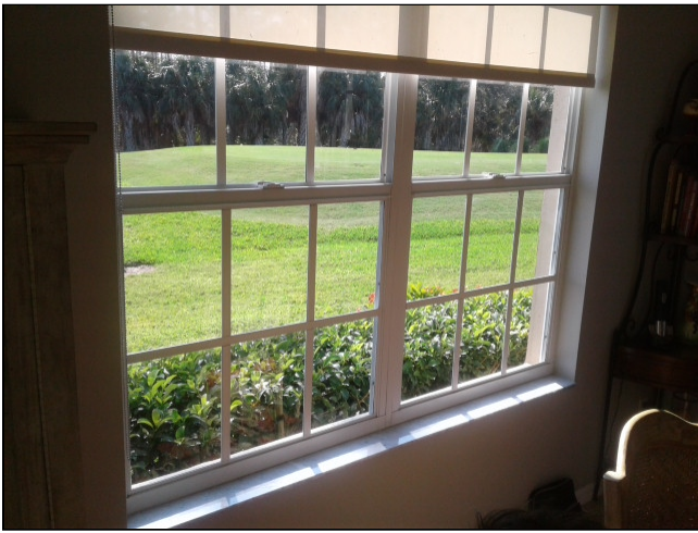
7.6.B Item 1(Picture) Rear windows without screens present (breakfast nook)
