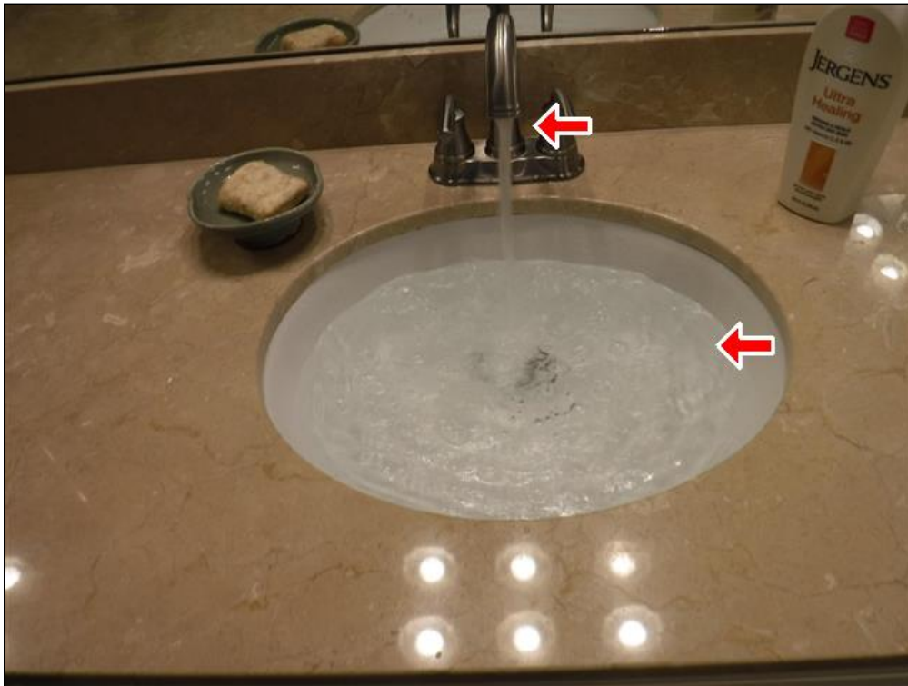
9.18.B Item 1(Picture) Missing aerator and slow draining
