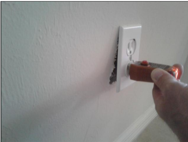
7.4.B Item 1(Picture) Broken outlet in living room
