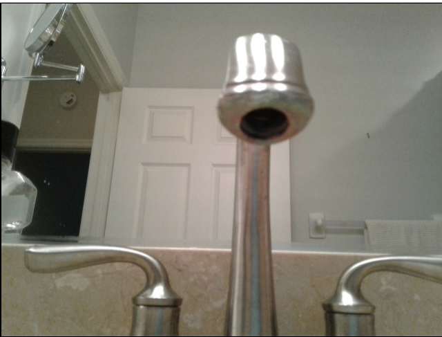
9.18.A Item 1(Picture) Sink faucet missing flow regulator screen
