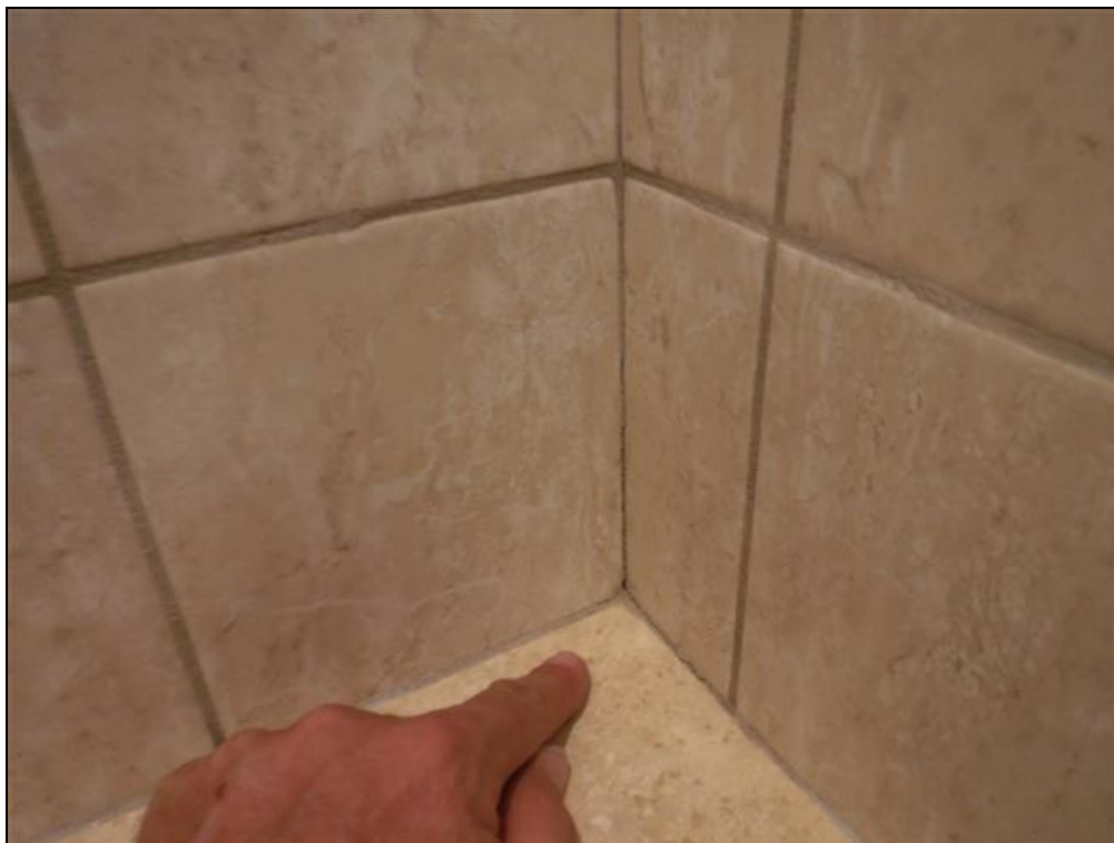
9.14.B Item 1(Picture) Minor grout cracks in corner
