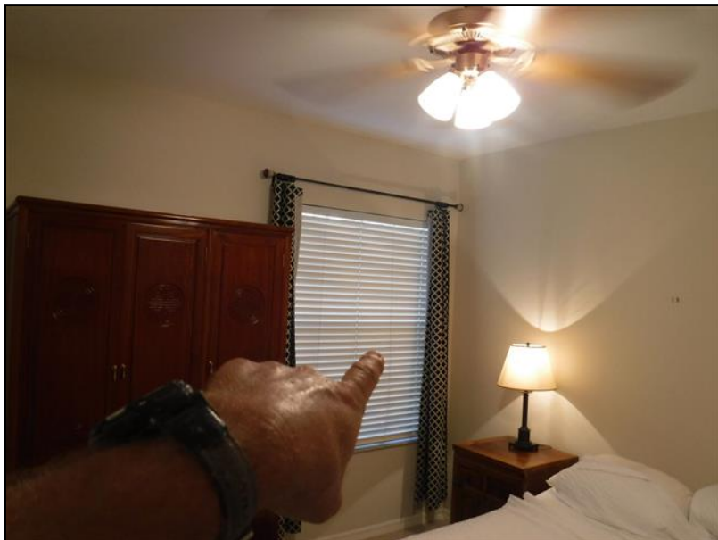
7.6.E Item 1(Picture) Front BDRM window not secured
