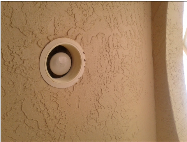
7.3.A Item 1(Picture) Front entry light not functioning (check bulb)
