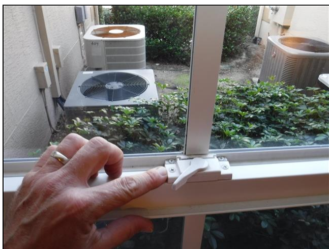
7.6.E Item 2(Picture) Locking not securing in window
