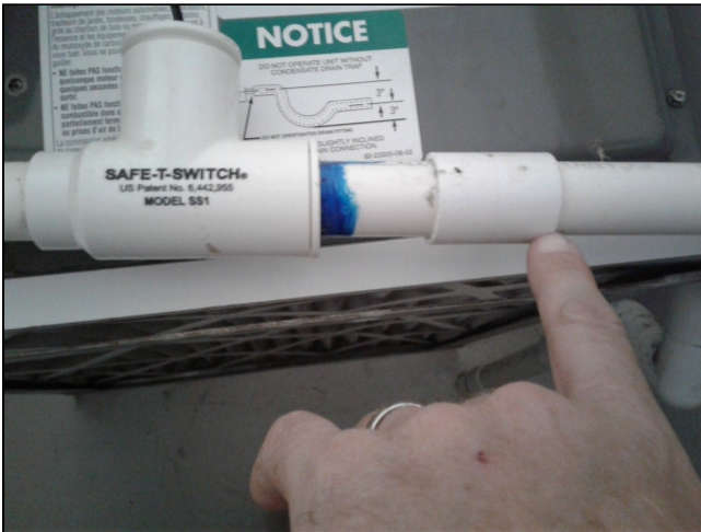
14.0 Item 1(Picture) Condensate line leaking at fitting(s)
