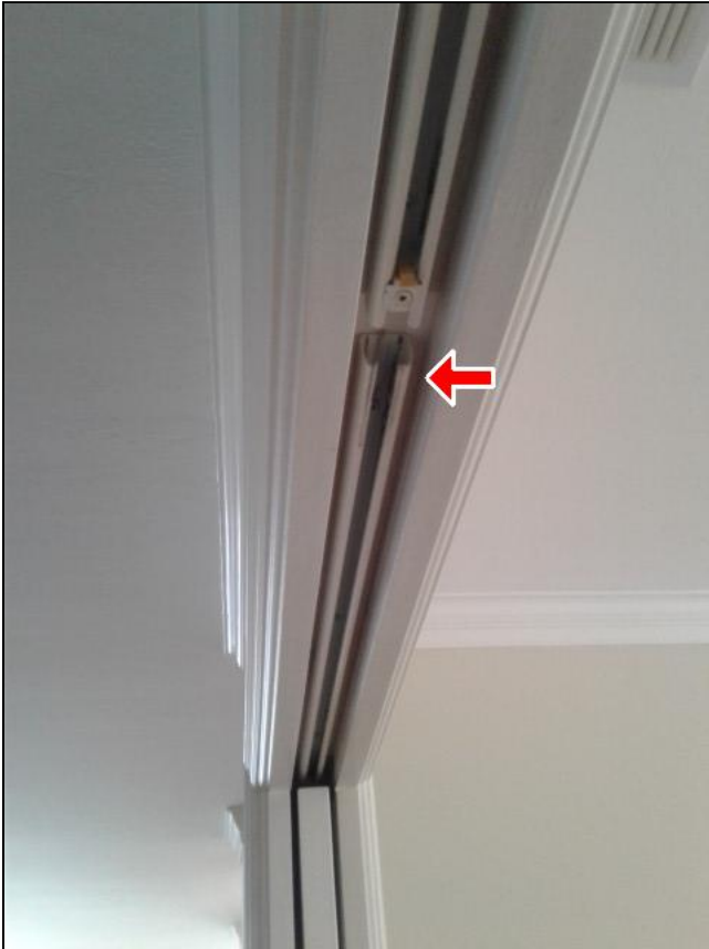
7.5.F Item 1(Picture) left side pocket door missing stop in overhead track
